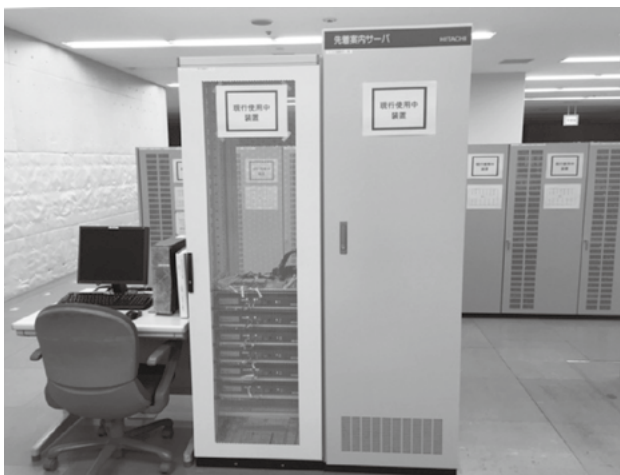
Fig. 3—Photo of the First-arriving Train Information Server and Monitoring/Input Terminals.
