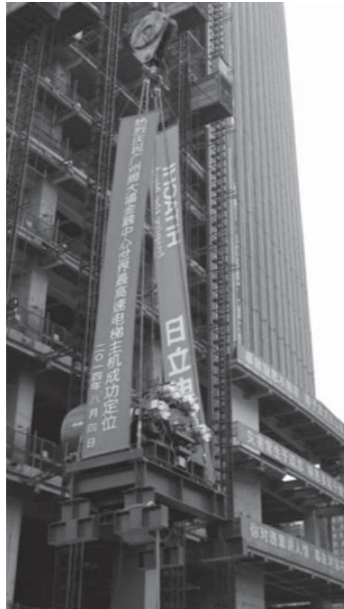
Fig. 17—Delivery of Fully Assembled Traction Machine. The photograph shows a traction machine and mount (with a combined weight of more than 20 t) being lifted up to the machine room after being assembled on the ground.
