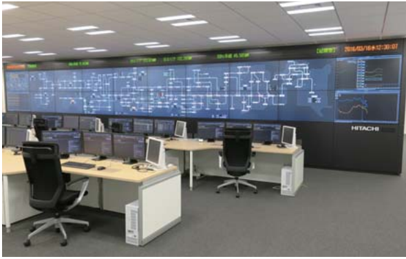
4 OCCTO operation center
