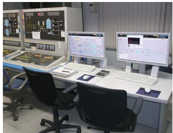
2 Central monitoring and control system for Yoshiba Purification Plant at Kuki City Waterworks and Sewage Department
