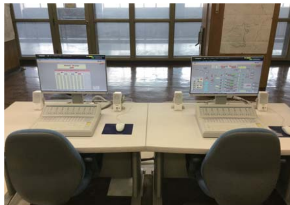
4 Monitoring office for Joto Distribution Plant at Osaka Municipal Waterworks Bureau
