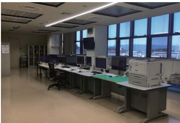
3 Central monitoring and control system for Nikko River Upstream Purification Center at Ichinomiya Construction Office, Aichi Prefecture
