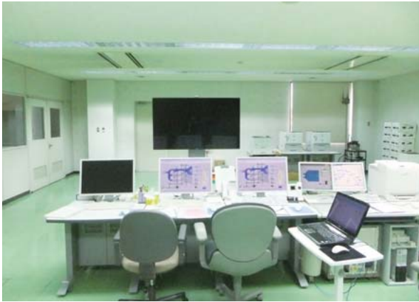
5 Monitoring and control system for Nuta River Purification Center, Hiroshima Prefecture
