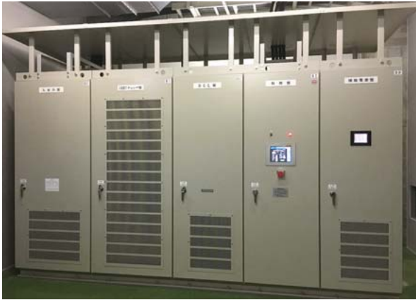
2 Stationary energy storage system chopper panel and new auxiliary power supply panel (far right)
