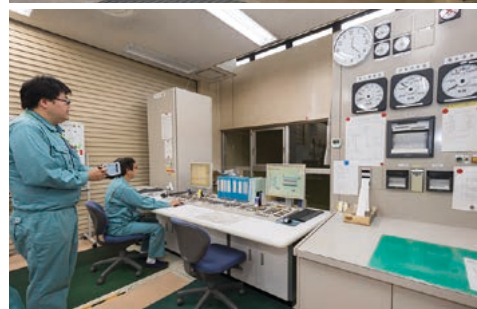
Niizo Pumping Station
