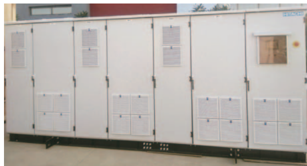
3 HIVERTER-NP215i Series of 1,500V DC-compatible solar PCS systems developed jointly with Hitachi Hi-Rel Power Electronics
