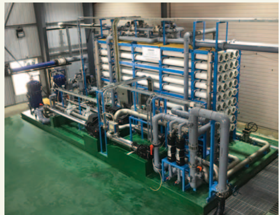
Figure 1 | Seawater Desalination Facility Delivered to Hulhumale Island, Maldives
